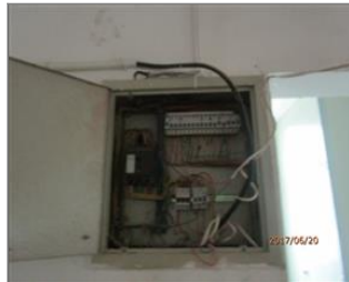
Photo of non-conformity 7.13 some switch boxes were opened and the switches were exposed outside.JPG
