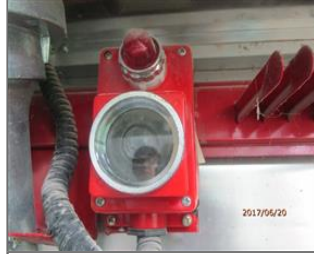
Photo of fire safety equipment Fire alarm.JPG
