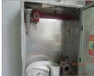
Photo of fire safety equipment Fire hydrant.JPG
