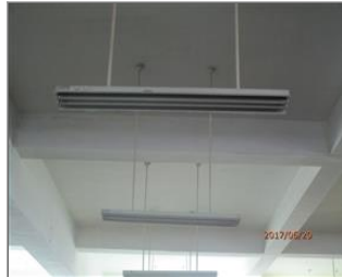
Photo of non-conformity 7.13 Normal fluorescent lamps without fire prevention measures of heat insulation and heat rejection.JPG
